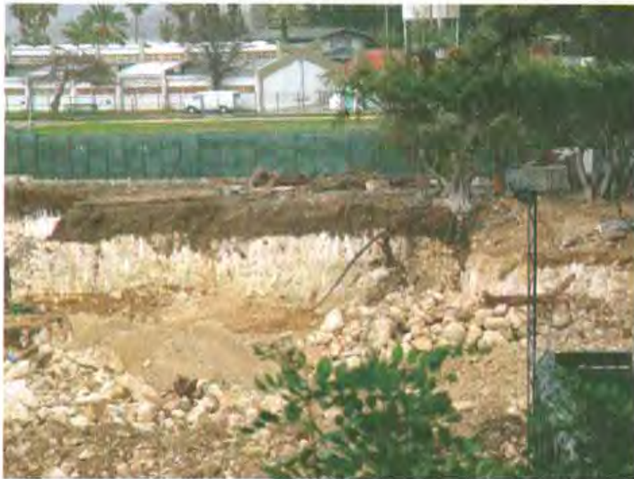
Fig. 9. This cross-section through the lower campus landscape during construction of the Charles W. Hostler Center shows the fertile soil (dark top layer), accumulated through decades of cultivation, above the limestone outcrop (light lower layer) (Photograph by the author)
